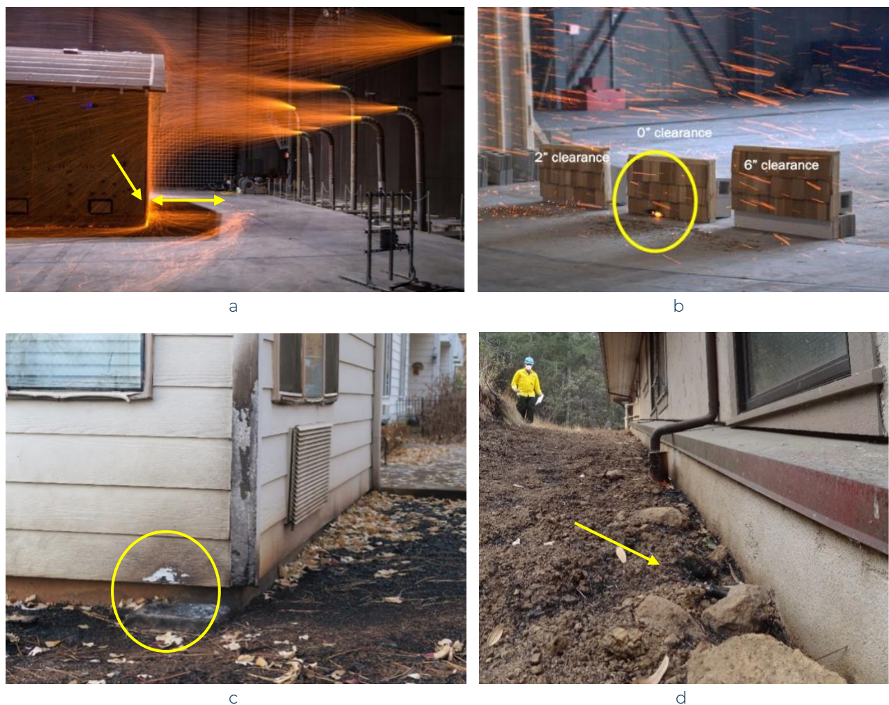
Figure 4. Ember accumulation at the base of the wall causing ignition (a and b) at the IBHS Research Center, (c) in the post-Camp Fire (2018) investigation in Butte County, California, and (d) at the base of a wall in the Glass Fire (2020) in Napa and Sonoma Counties, California, which did not have the opportunity to grow because of a noncombustible vertical clearance.
